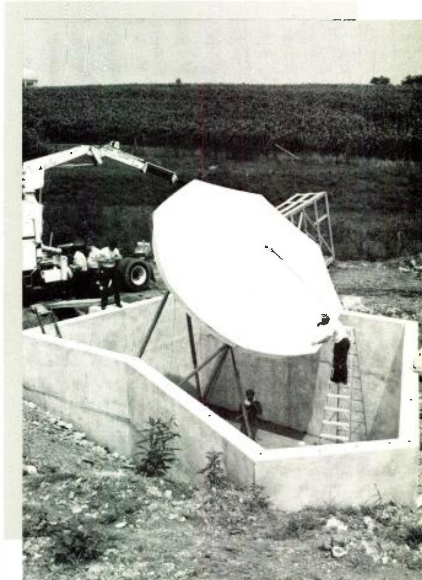
Showing one way to reduce interference from terrestrial signals, antenna at WEKU, Richmond, KY was installed in pit.
